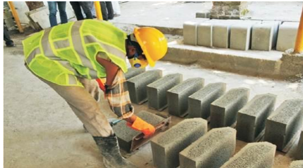
Kerb Stones made with LC 3 - Jhansi
